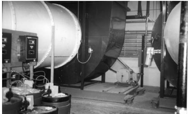
Figure 5. Fan mounted on an inertia base
