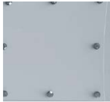
Bolted Inspection Door
