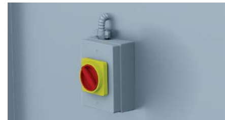
NEMA 4 Disconnect Switch
