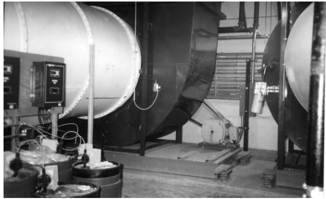
Figure 5. Fan mounted on an inertia base
