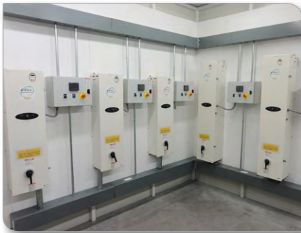
Explosion-Proof Control Room
